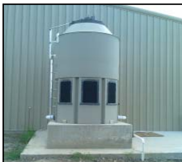
Example of locally installed cooler
