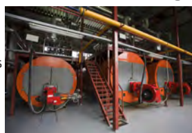
Boilers & Process Heat
